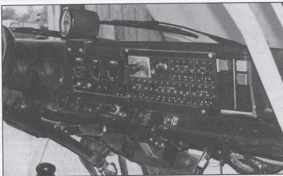
The circuit breaker panel allows the co-driver easy access to identify and correct any on-board electrical problems.
