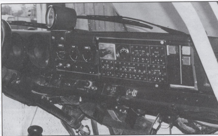
The circuit breaker panel allows the co-driver easy access to identify and correct any on-board electrical problems.
